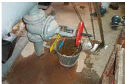
Condensate leakage (Photo: J. Burjaniv)
