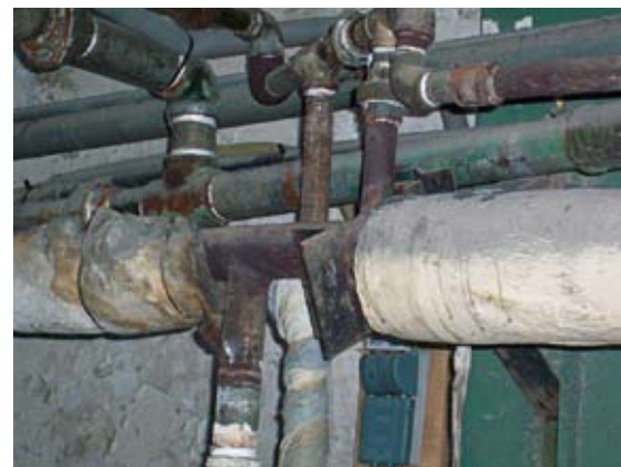
Wrong pipelines installation and insulation
