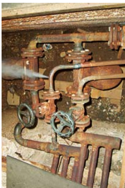
Steam leakage (Photo: J. Burjaniv)
