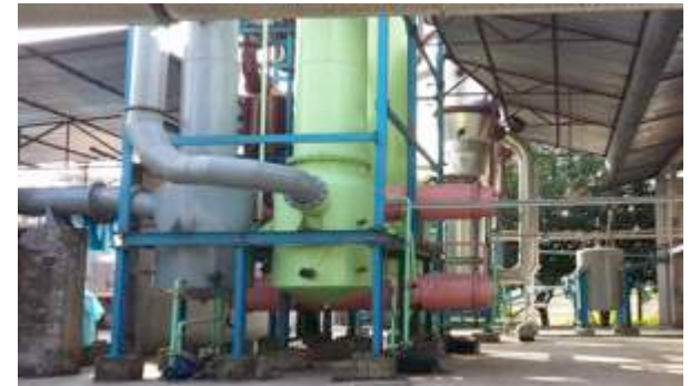
Financed 1 Biomass Based Power Projects
