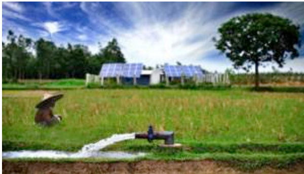
602 Solar Irrigation Pumps in Operation
