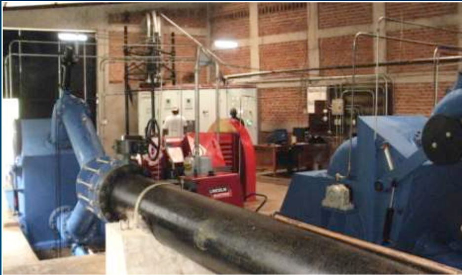
El Bote powerhouse 900 kw two pelton turbines
