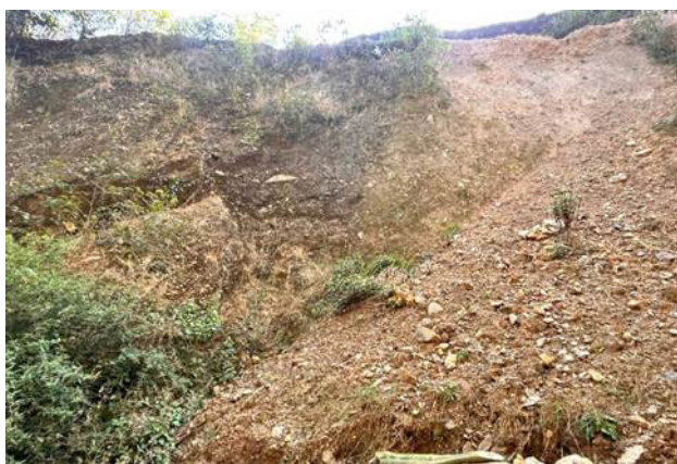
Slope adjacent to the road above the powerhouse and the channels before intervention
